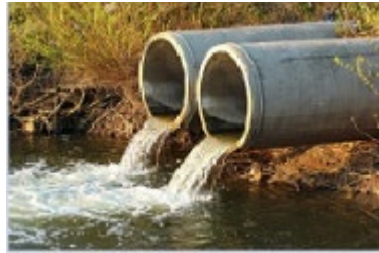
Drainage facility UGD
